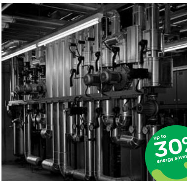
ATV12 drive controlling a pumping station
