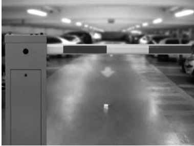
ATV12 drive controlling an access barrier
