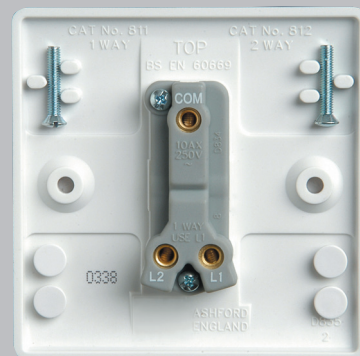
All light switches 10AX rated
