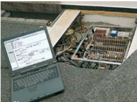
Floor distribution boxes
