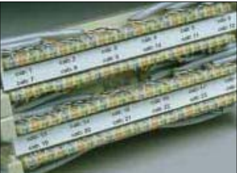
Network Systems Labeling
