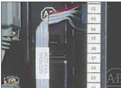
Terminal Block Labeling
