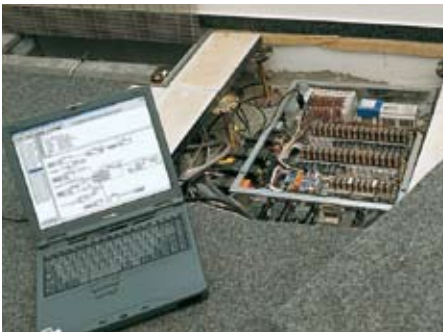
Floor distribution boxes
