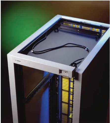
Rack with PDU and switch
