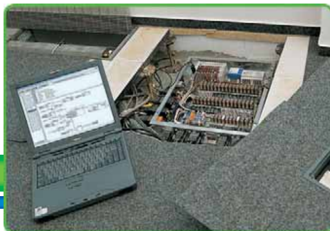
Under-floor distribution boxes
