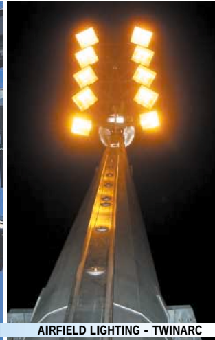
AIRFIELD LIGHTING - TWINARC
