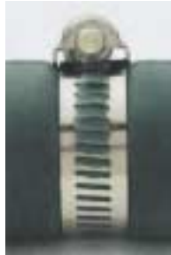
Hose installed with unlined clamp
