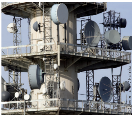
Telecom - Data infrastructure
