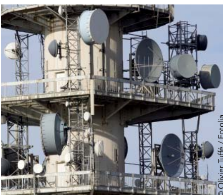
Telecom - Data infrastructure
