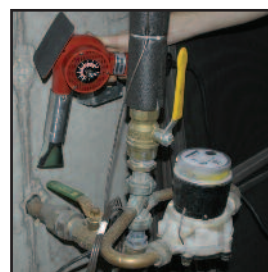
Thaw Frozen Pipes
