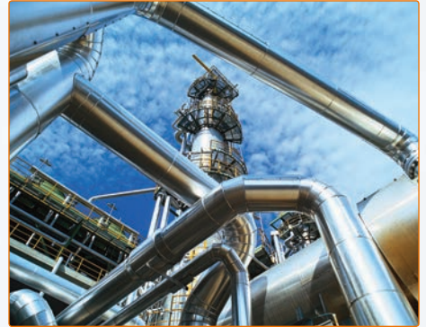
Chemical, Oil and Gas
