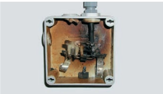
Module box after lightning strike
