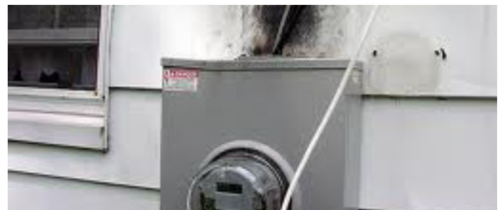
Service entrance destroyed by a surge
