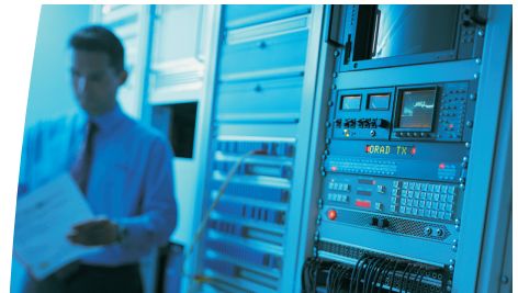
Servers, data storage and network equipment.
