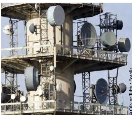
Telecom - Data infrastructure
