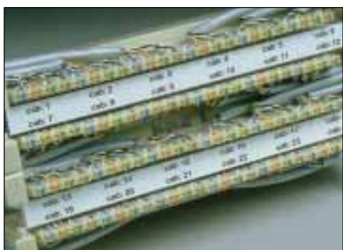
Network Systems Labeling
