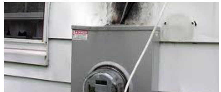
Service entrance destroyed by a surge
