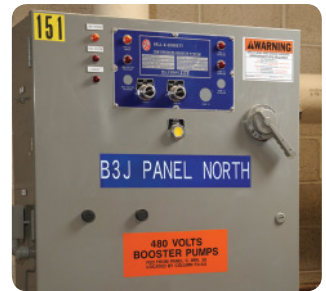
Control Panel & Electrical Panel Labels
