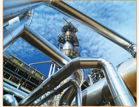
Chemical, Oil and Gas
