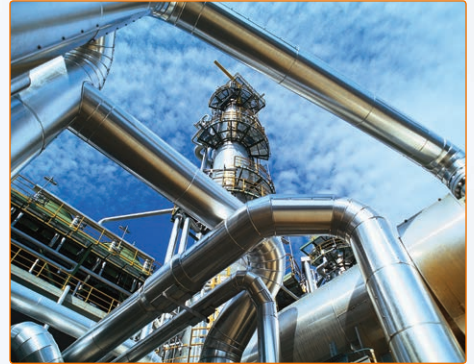
Chemical, Oil and Gas
