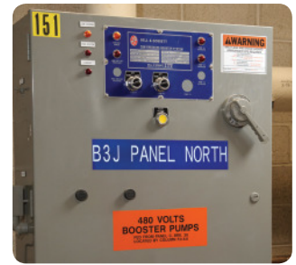
Control Panel & Electrical Panel Labels
