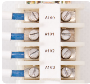
Terminal Block Markers
