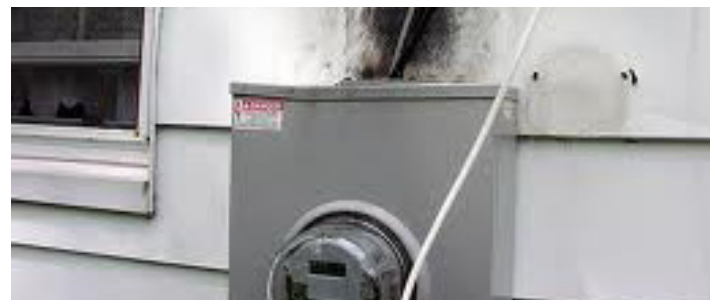
Service entrance destroyed by a surge
