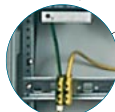
Surge arrester / Earth terminal
