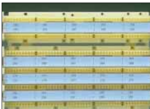
Network Systems Labeling
