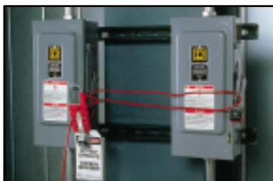
Lockout Single or Multiple Disconnects
