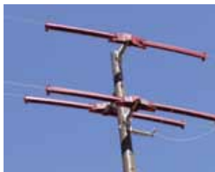
2 Pieces: MVLC-38 on busbar with BCIC
