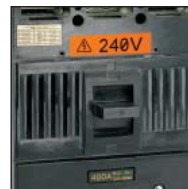
Electrical Hazard Labels
