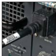
Electrical Infrastructure Labeling
