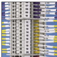
Terminal Block Labeling
