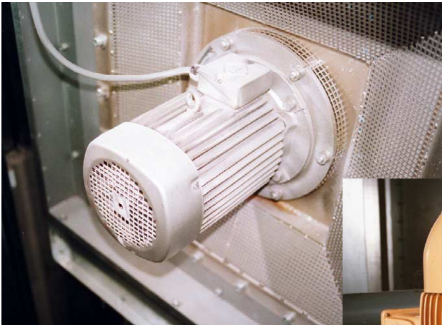
Monitoring a motor in a cooling system
