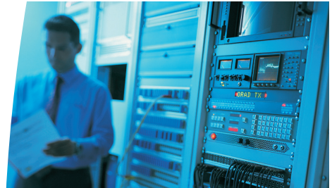
Servers, data storage and network equipment.
