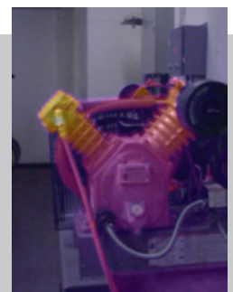
Air Compressor – AutoBlend™ Mode
