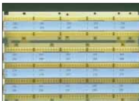
Network Systems Labeling
