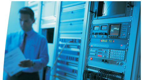
Servers, data storage and network equipment.
