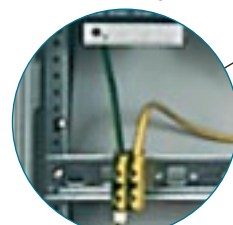
Surge arrester / Earth terminal
