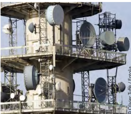
Telecom - Data infrastructure
