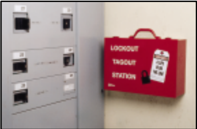
Mount close to power and distribution panels
