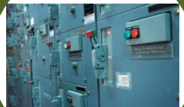
Industrial Control Panels
